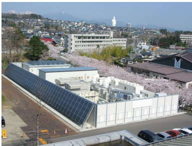
Figure 1: Sendai Microgrid in Japan ( https://building-microgrid.lbl.gov/sendai-microgrid ).
